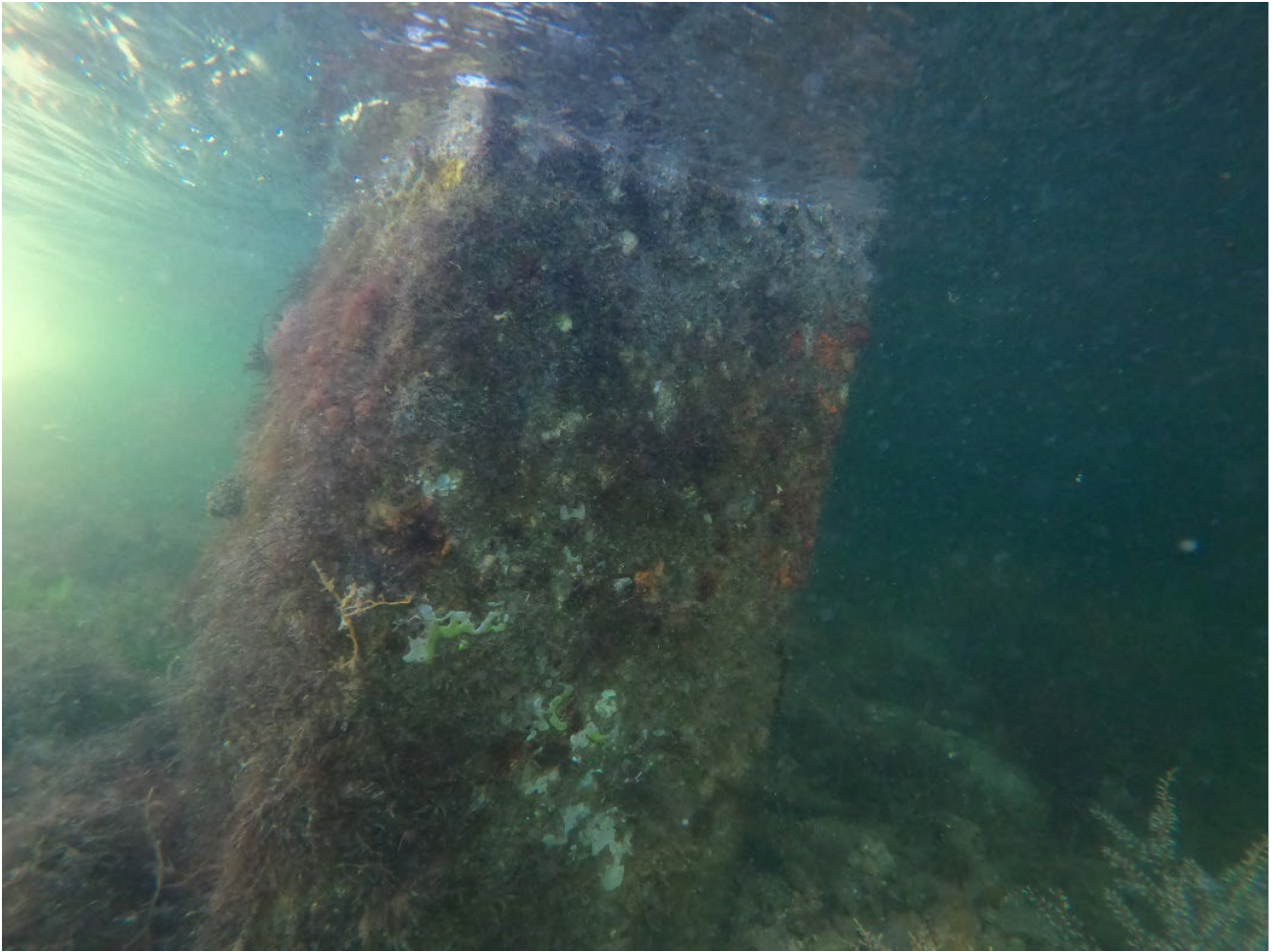
Photo 13 Dense coverage by sponges, octocorals, and tunicates observed on bridge pilings in the photic zone on the south side of the eastern bridges (typical).
