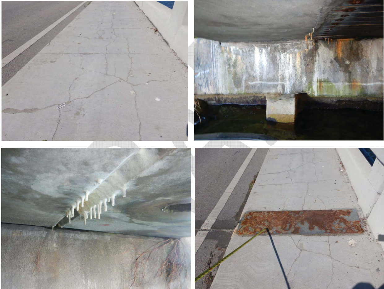
Figure 2.2 | Representative Photos of Damage at Bridge 870083 (October 2020)
