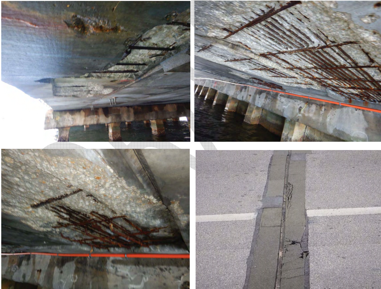
Figure 2.3 | Representative Photos of Damage at Bridge 870084 (October 2020)
