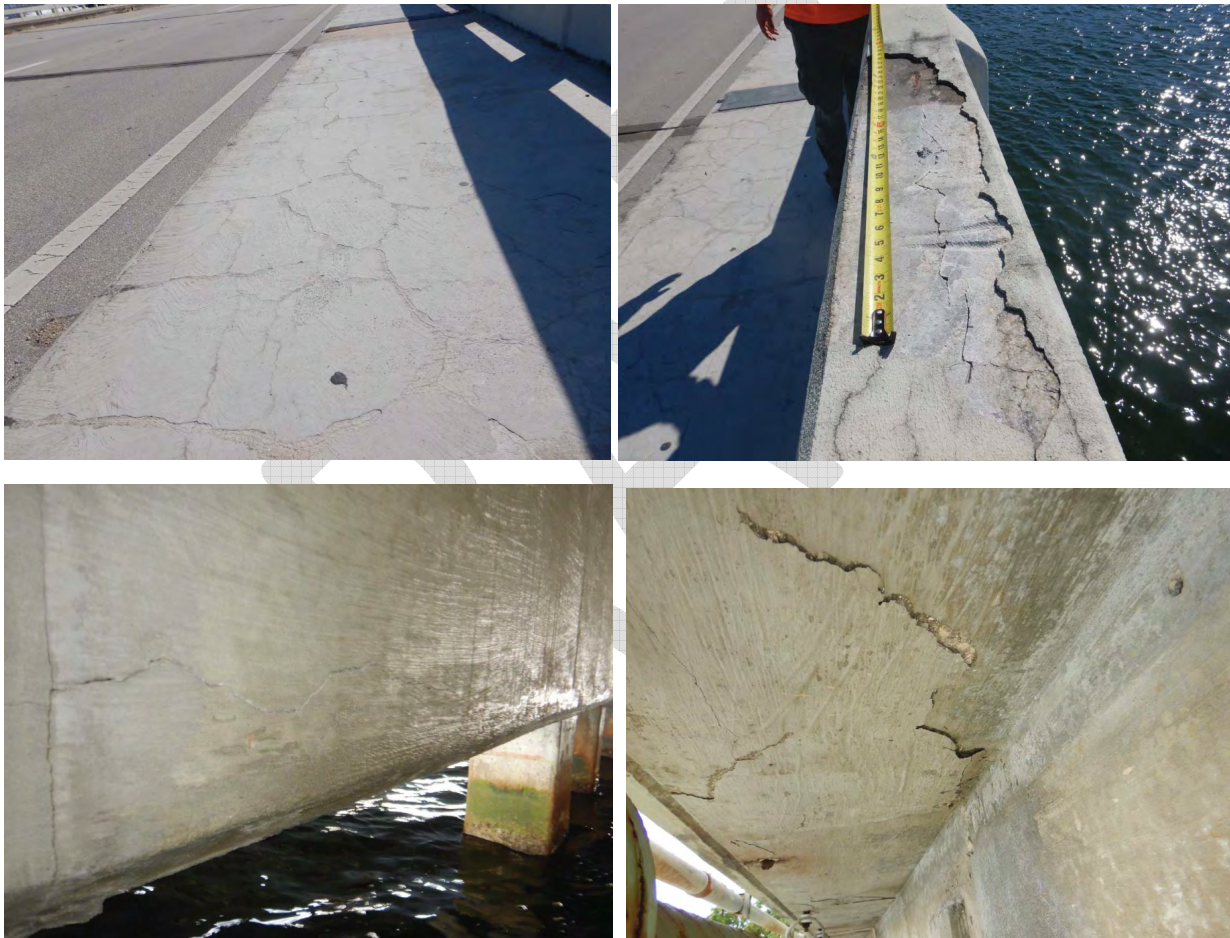
Figure 2.4 | Representative Photos of Damage at Bridge 870549 (October 2020)
