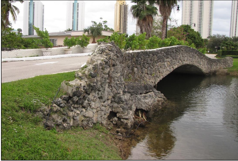
Figure 2: Exterior Surface and Low Arch of Atlantic Island Bridge/FDOT Bridge No. 874218 (8DA6433), Facing Southeast
