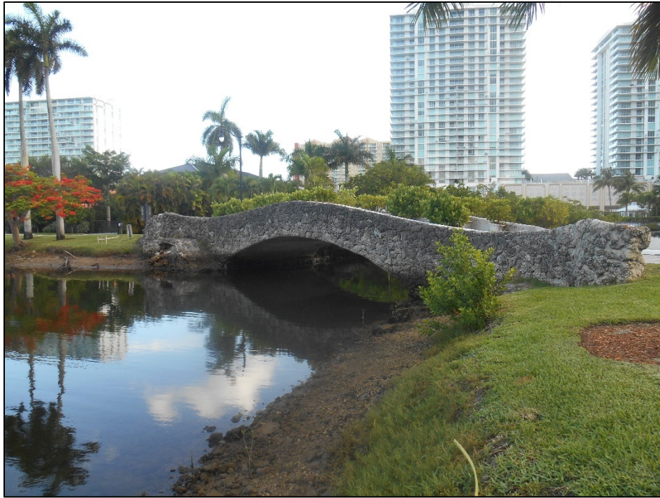
Figure 3: The Atlantic Island Resource Group (8DA15825), contains the Atlantic Island Bridge (8DA6433), Lake of the Isles (8DA15824) and Atlantic Island Park (8DA15825), c. 1925, considered National Register-eligible, facing East
