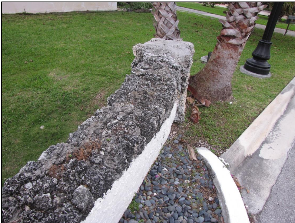
Figure 4: Whitewashed Stucco at Interior of Railings of Atlantic Island Bridge/FDOT Bridge No. 874218 (8DA6433), Facing Southeast
