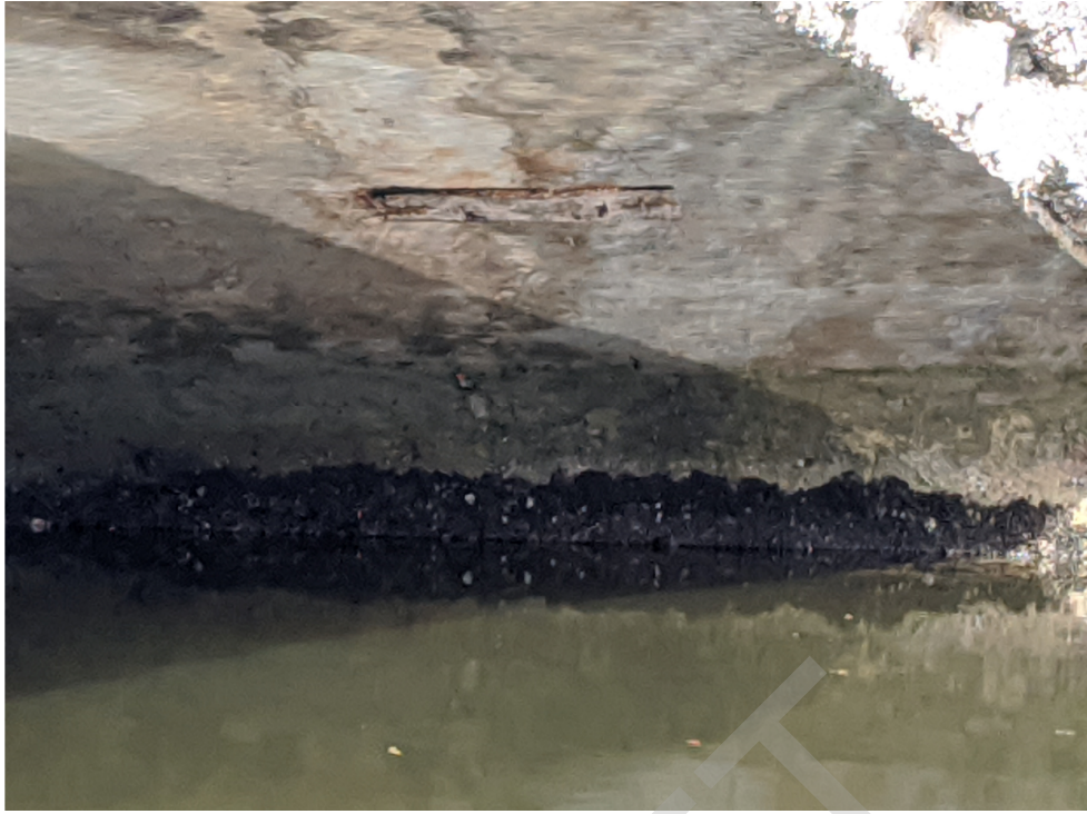
Figure 23: Damaged Stucco at Underside of Bridge Covered with Wooden Plank – Looking East
