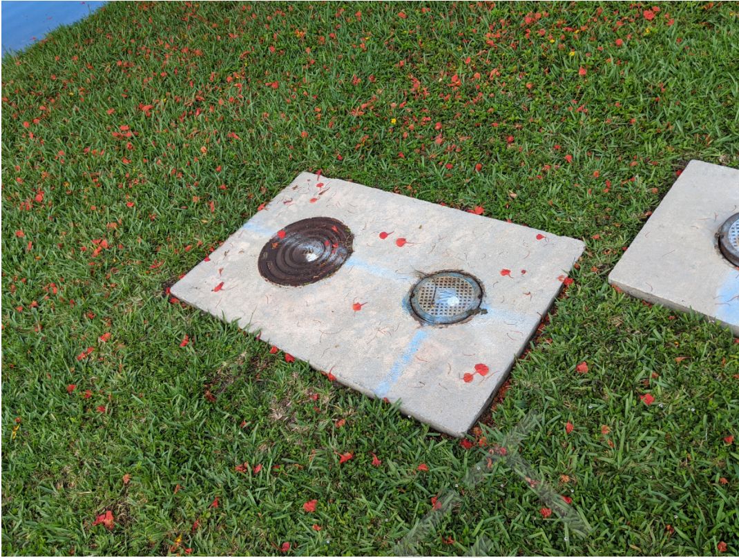
Figure 11: Water Valves – SW Corner (2 of 2)
