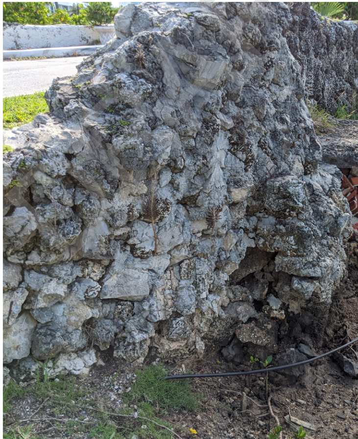
Figure 22: Coquina Limestone Rubble Attached to End of Parapet – SW Corner (2 of 2)
