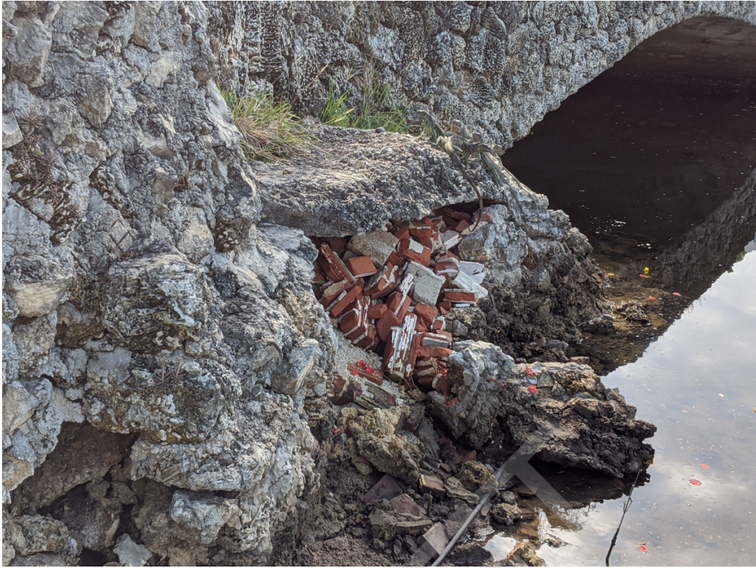
Figure 15: Damage to Western Abutment – Looking NE
