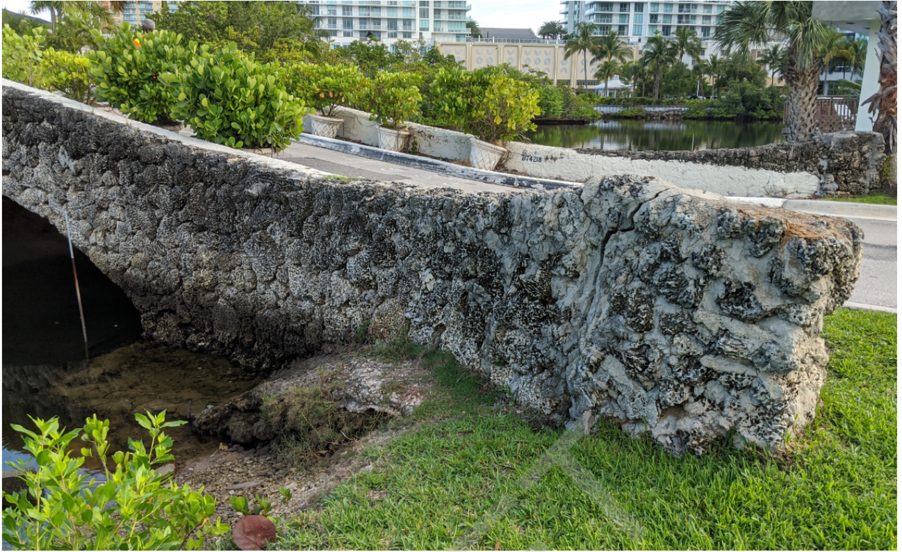
Figure 19: Cracked Coquina Limestone Rubble Attached to End of Parapet – SE Corner (2 of 2)
