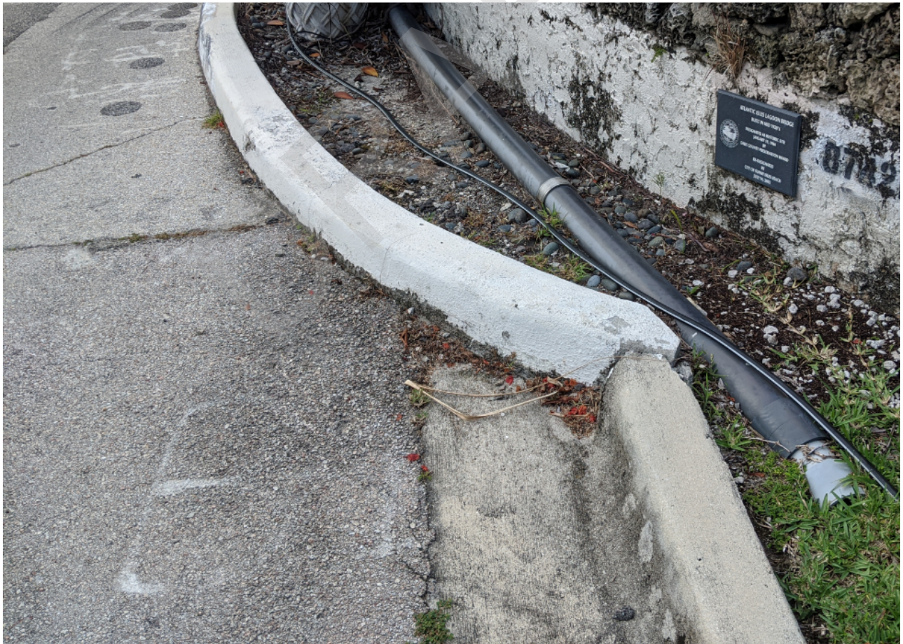
Figure 8: Utility Pipe (8" Diameter Water PVC) Along Southern Planter
