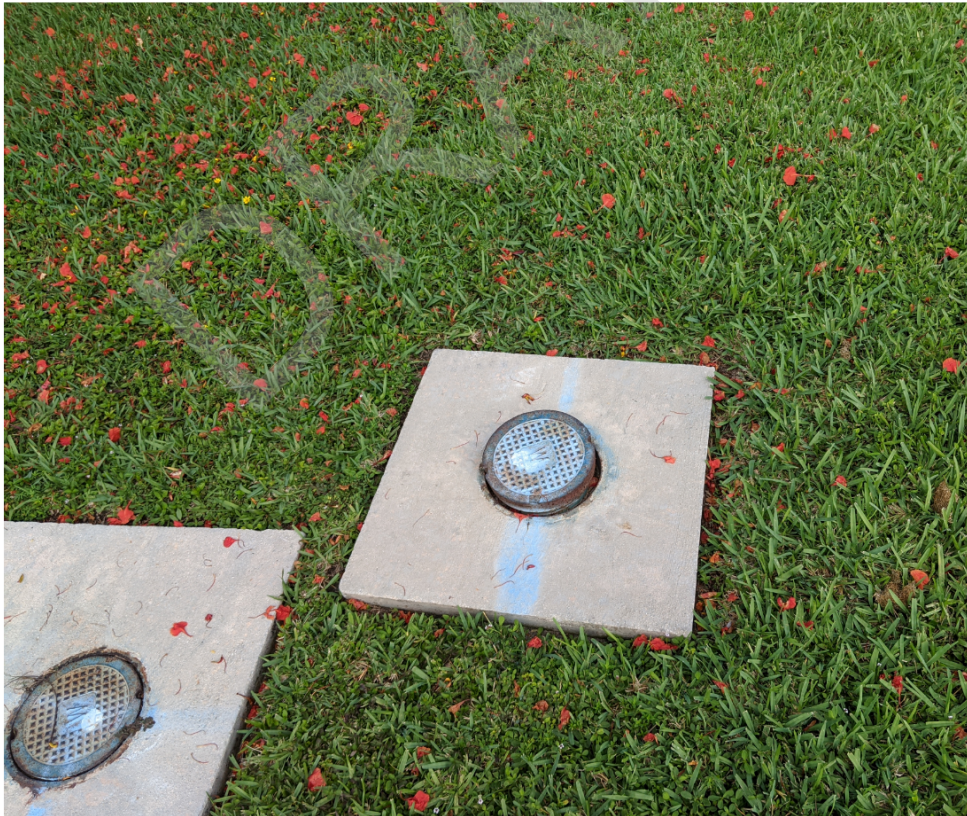
Figure 10: Water Valves – SW Corner (1 of 2)
