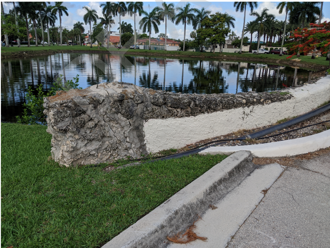
Figure 18: Cracked Coquina Limestone Rubble Attached to End of Parapet – SE Corner (1 of 2)
