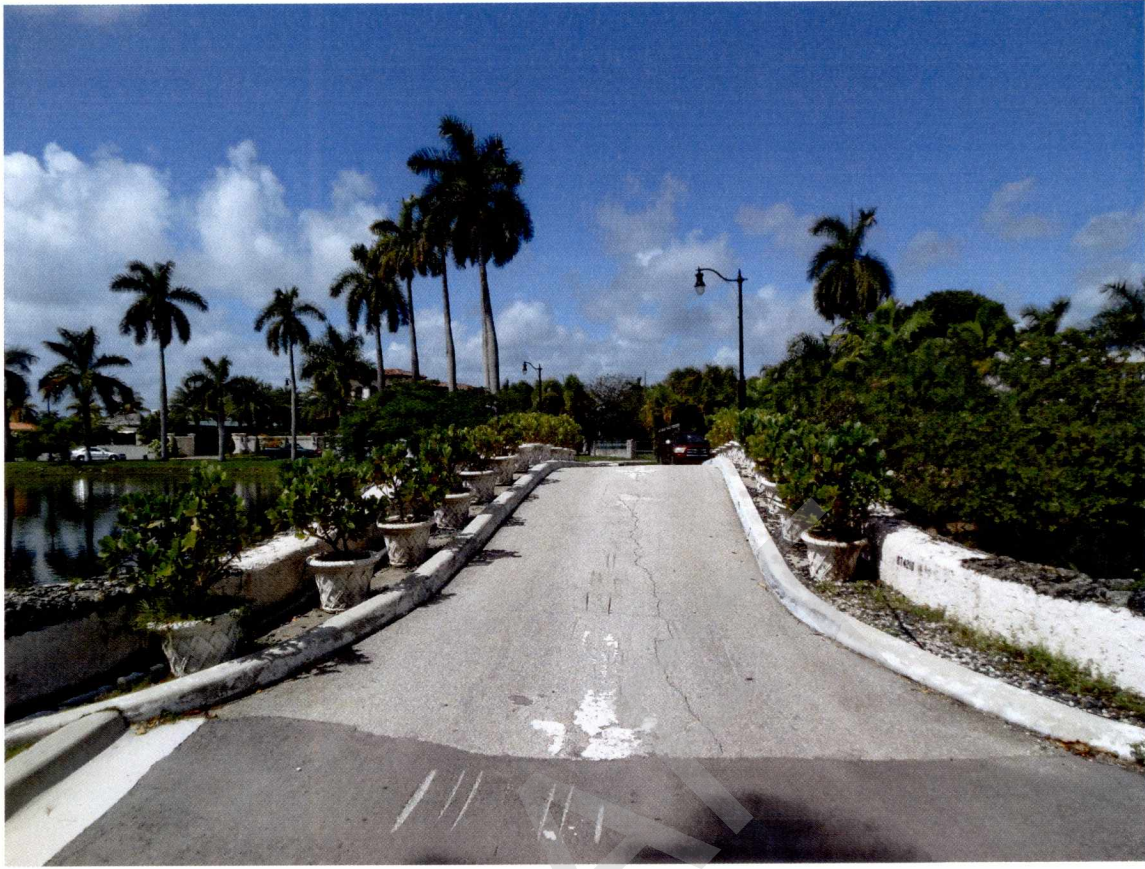
Longitudinal crack through asphalt on Bridge
