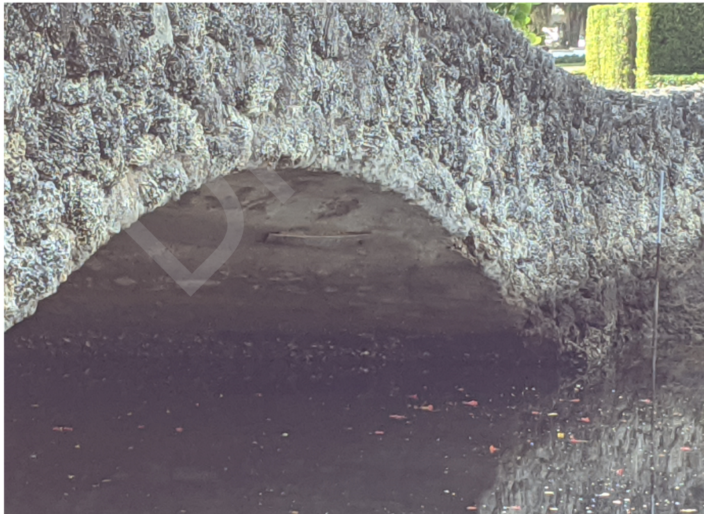
Figure 24: Damaged Stucco at Underside of Bridge Covered with Wooden Plank – Looking West
