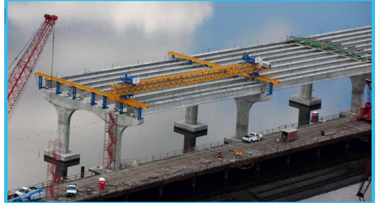
Lateral beam shifter will be utilized to set girders into their final position without the need for dual cranes on the deck. This system was used by Archer Western on FDOT D4's Award Winning Veterans Memorial project.
